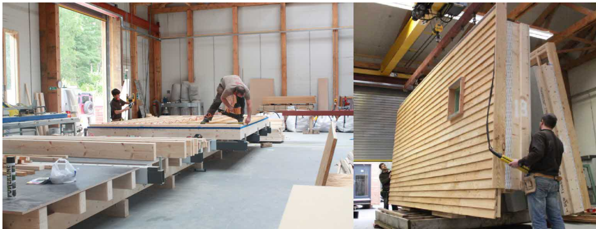
MAKAR Workshop, Inverness (above), and typical off-site constructed wall panel being craned into place on site (below)
